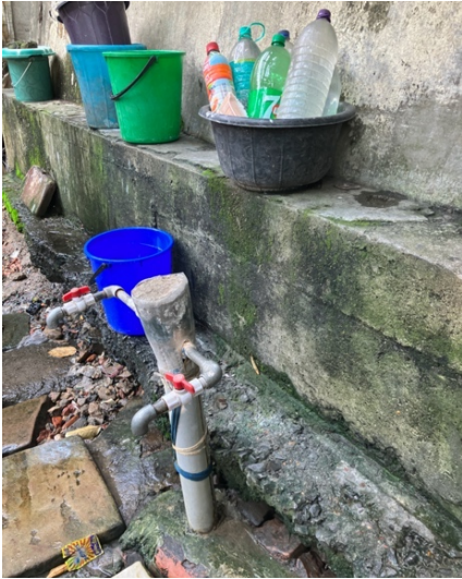
A crucial improvement: There is now a public water tap that is open twice a day. An important contribution to health in the slum.
